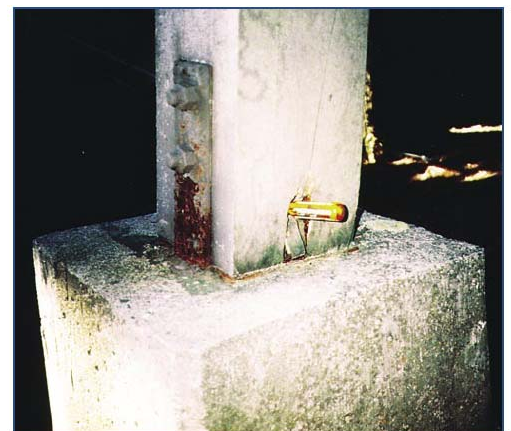
Wood decay at the base of a wood post supported by concrete.
